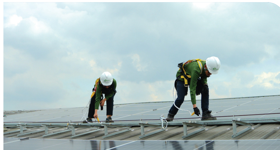
HIJAU's engineers perform on-site inspection and routine monitoring of the rooftop solar PV system by adhering to proper PPE usage and safety procedures.
