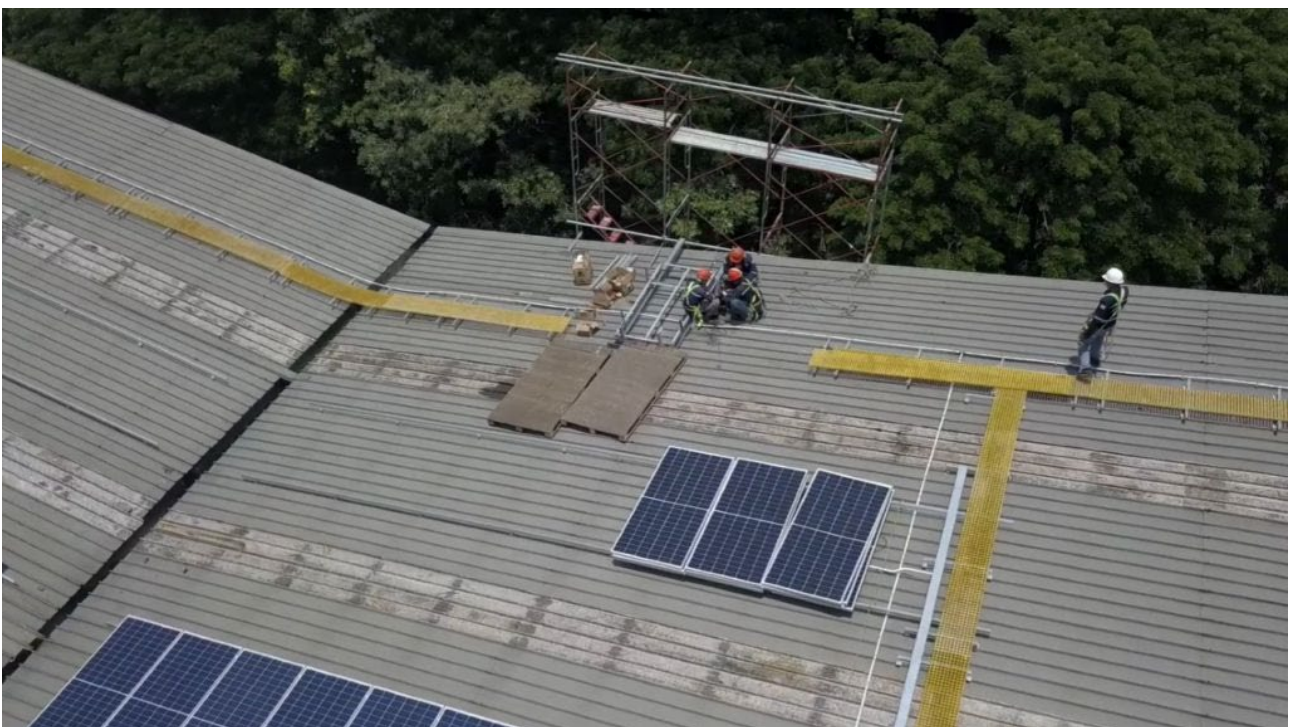
Image: Xurya solar installation, Indonesia
